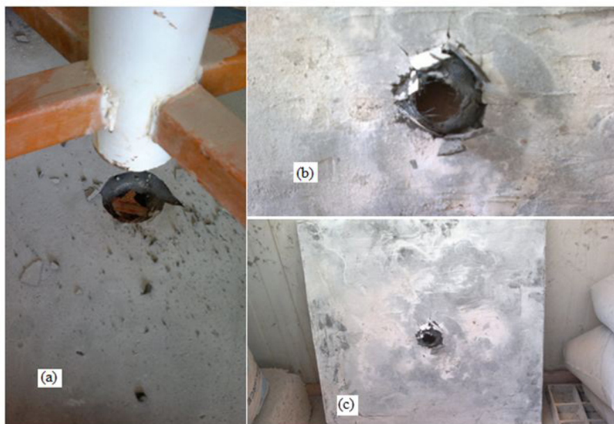
Photo 1(a-c): The damage of the nano ferrocement plates was generally local
